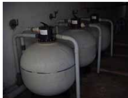
Figure 5: pressurized sand filters
