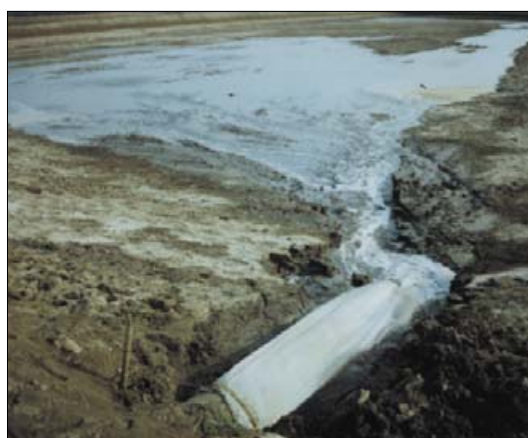
Water filtration using single bag filter
